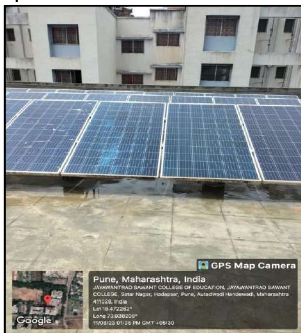
Photograph of Roof Top Solar PV Plant:
